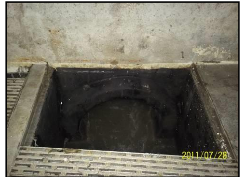
30-inch influent Pipe
