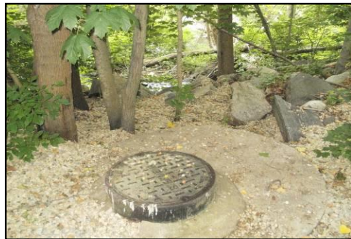
Pump Station Influent Manhole
