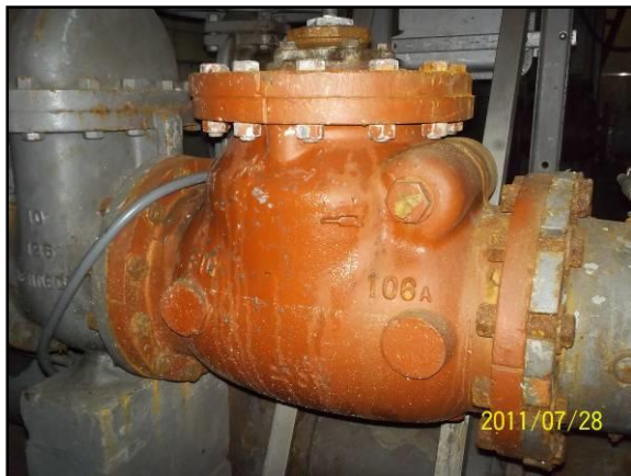
10-inch Check Valve on Discharge Line
