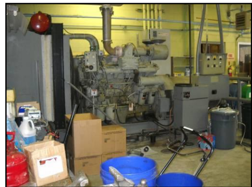
350 kW Emergency Generator
