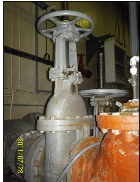
10-inch Gate Valve on Discharge Line
