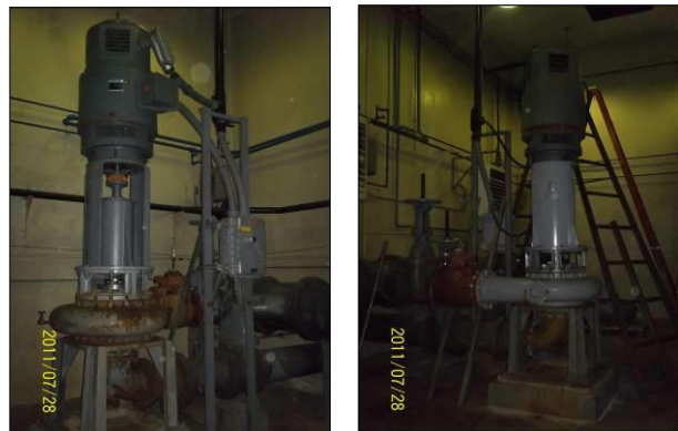
Existing Pumps No. 1 (Left) and No. 2 (Right)
