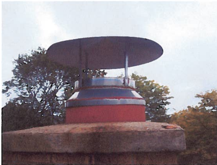
Photo 4: Waterproof concrete chimney cap with fluid applied flashing specified in section 07555. Extend flashing to top edge of clay chimney.
