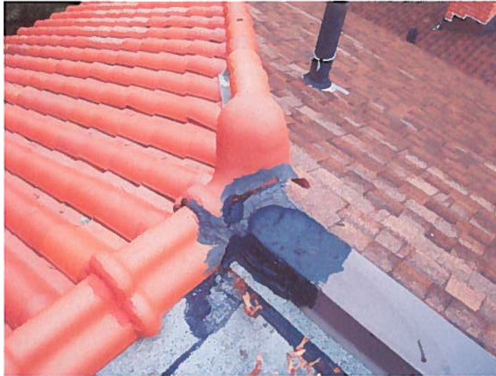
Photo 3: Replace broken cap tiles here and elsewhere.
